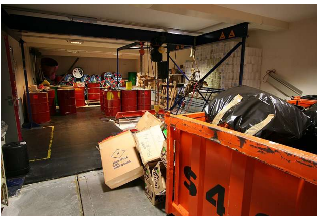
The waste-room at SANAE IV - containers with bales of paper/plastic waste and cardboard are visible on the right, while the drums used for other waste are visible to the top left.
